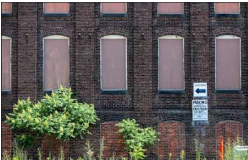
The site of the defunct Hampden Papers Inc. at 100 Water St. in Holyoke, where the Boston based Chestnut River Power and Infrastructure is proposing the construction of a $200 million data center. (Michael J. Fiedler / Special to The Republican)Michael J. Fiedler / Special to The Republican
